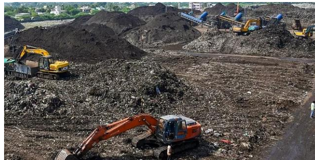
Figure 14-20: Existing situation of Ariyamangalam Dump Yard
