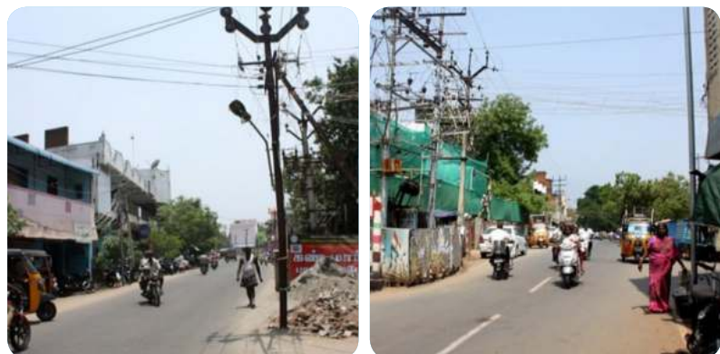
Fig 7.3: Light Poles and Transformer in RoW
