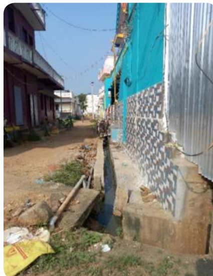
Fig 8.7: Sullage in Open Drains in Non-Municipal Area (Sholapuram Village)
