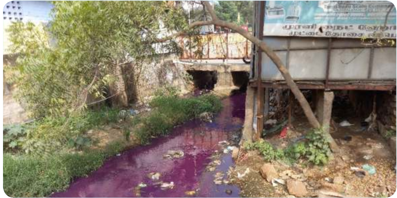
Fig 8.23: Encroachment on Storm Water Drain which is Polluted in Municipal Area
